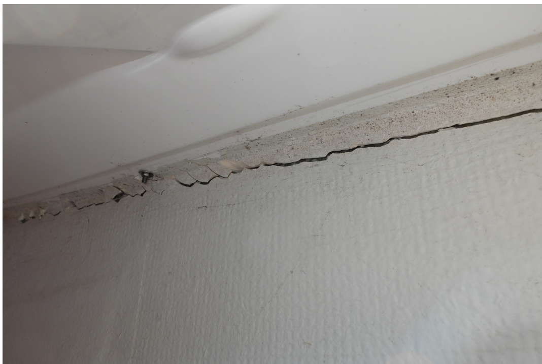
Photo Marcel Arditì: Mamma Mia's crack caused by a speeding water-skiing motor-boat
